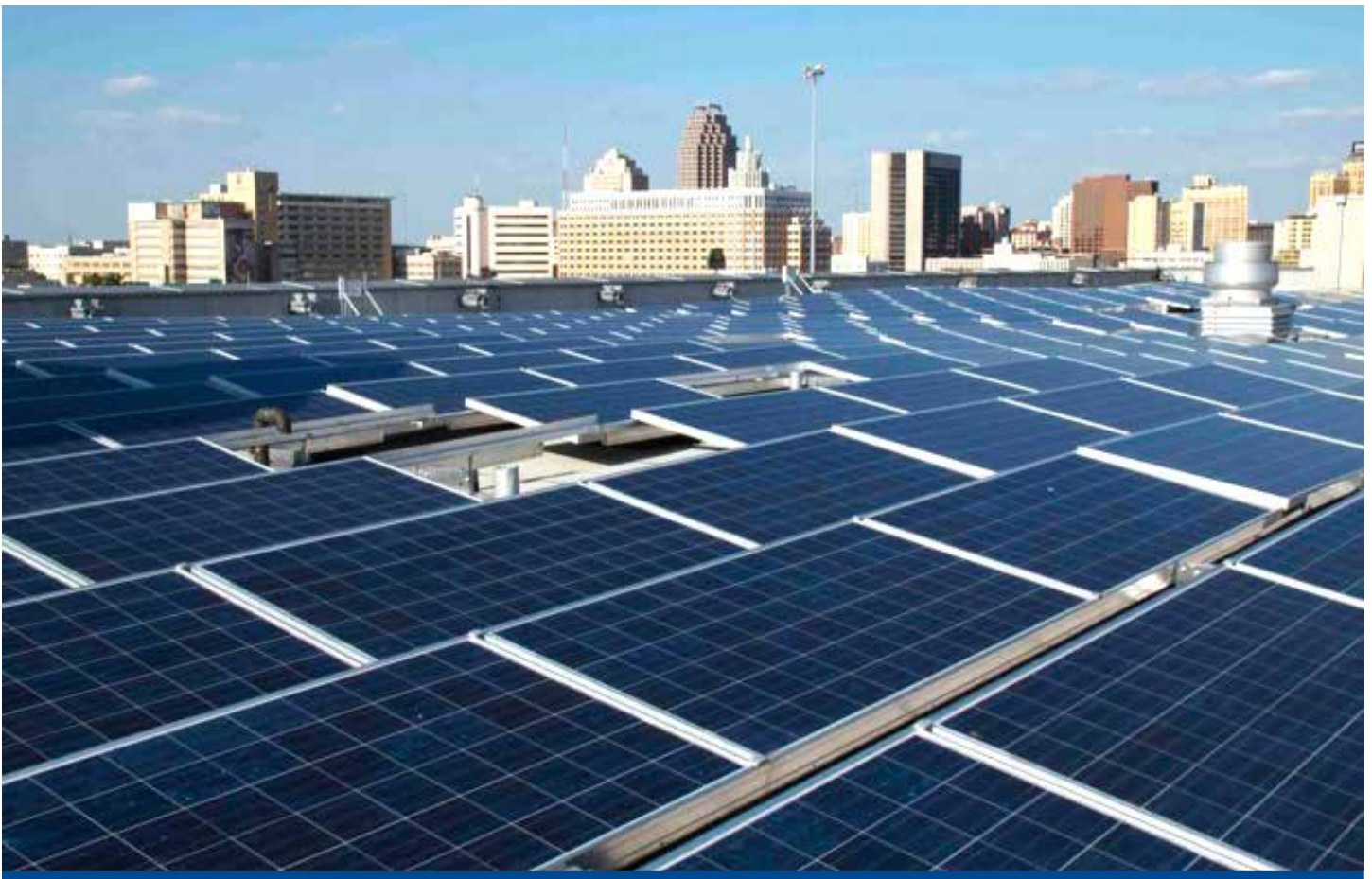
The San Antonio skyline beyond rows of solar panels.
